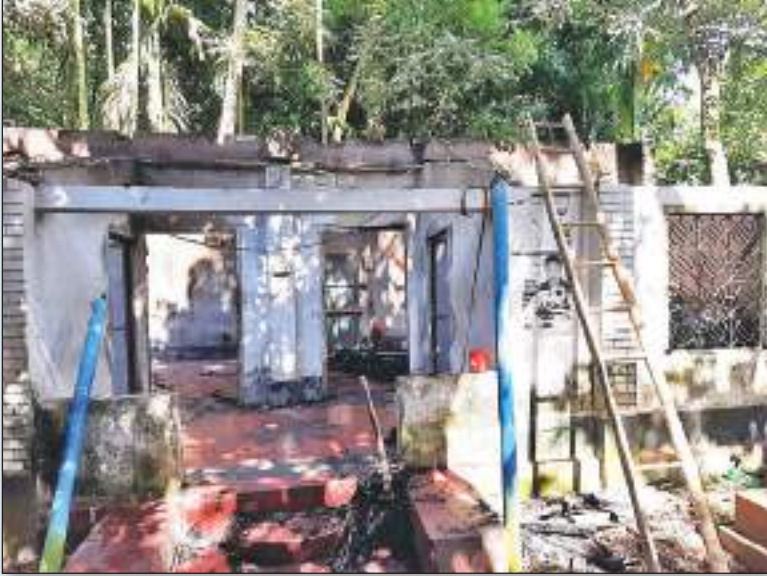
Vandalized houses in Narail (Source: Prothom Alo)
